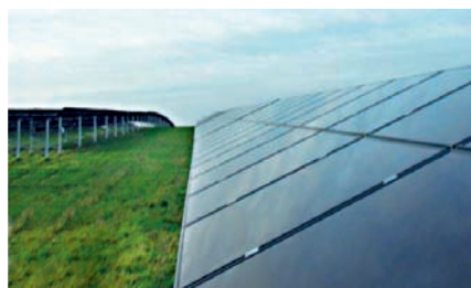
Solarpark Blankenberg, 1.109 kWp
