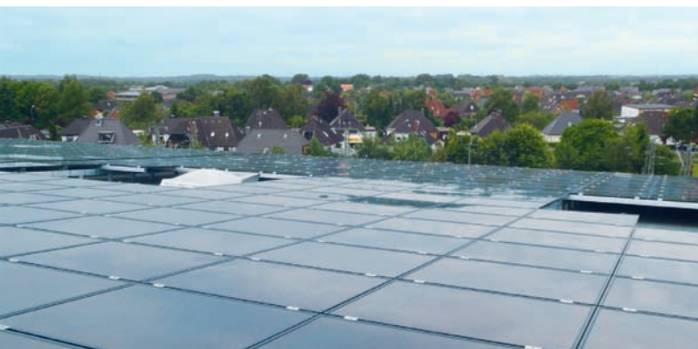
Photovoltaik-Dachanlage, Spedition in Handewitt
